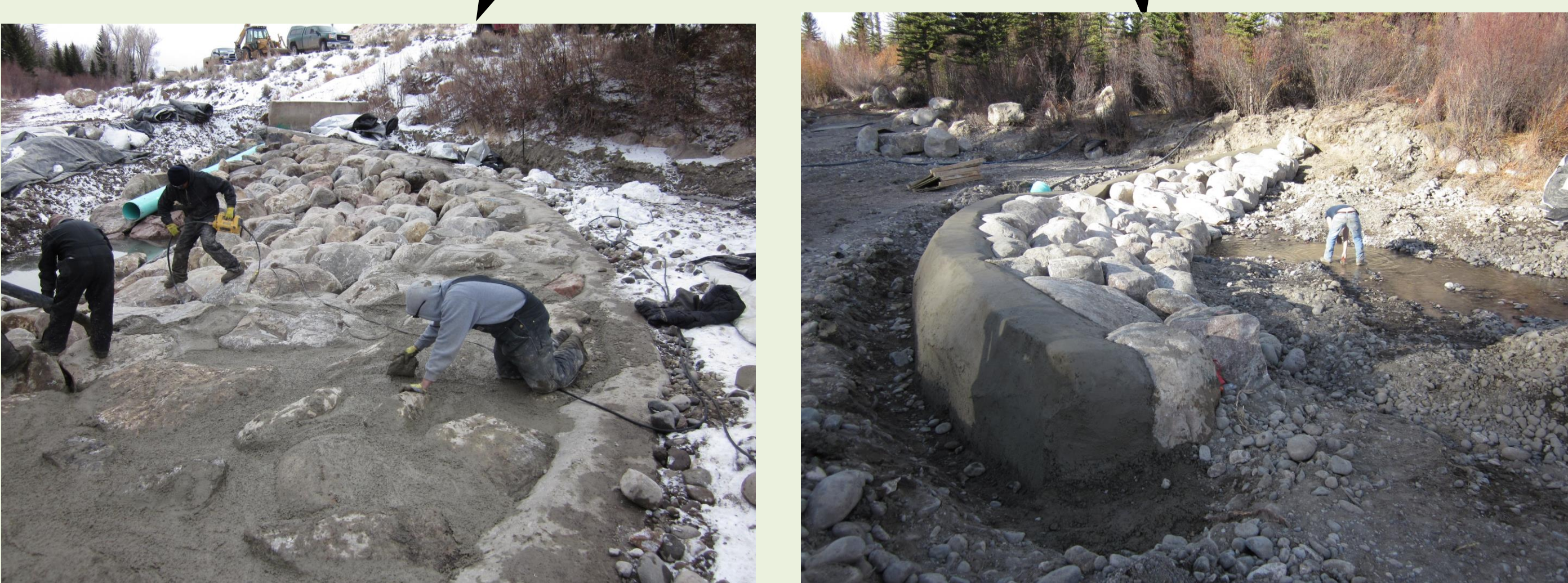
Upper grouted vane looking towards headgate. Teal pipe is the sluiceway
