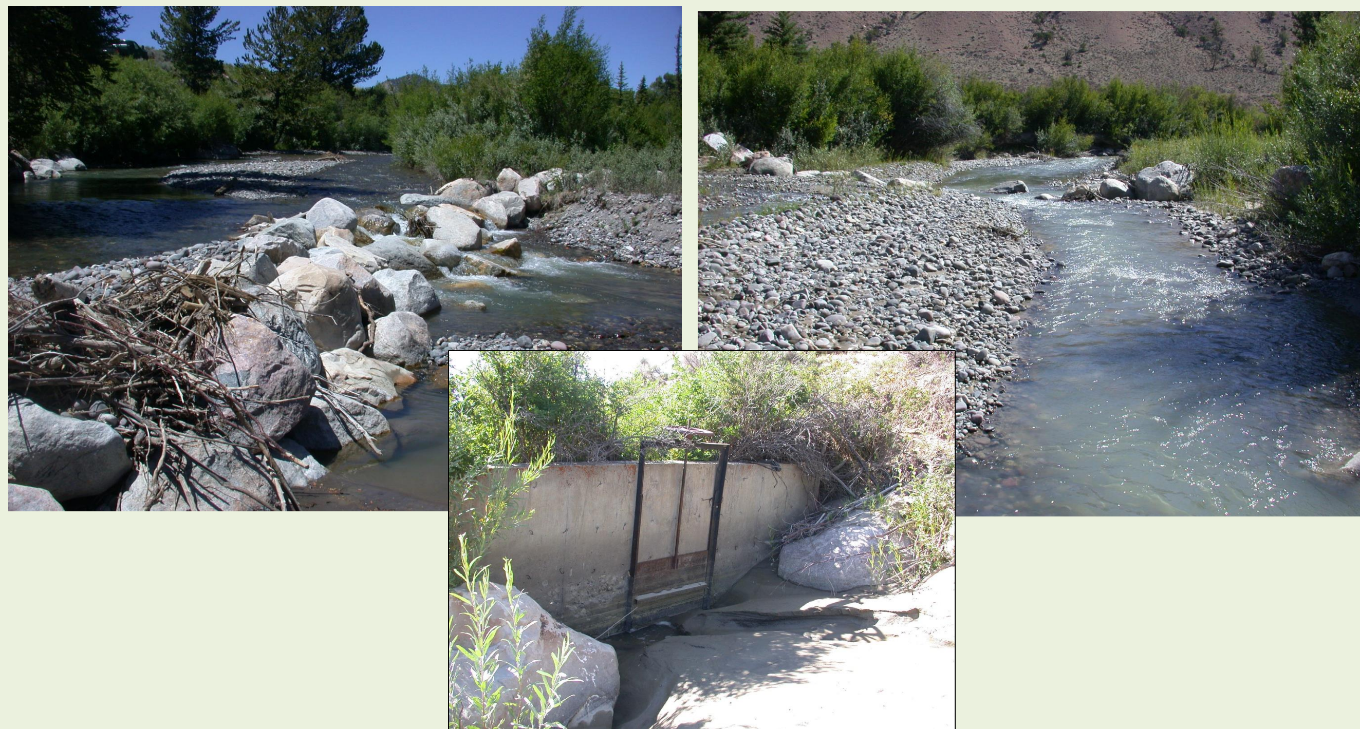
Figure 2. 2010 conditions of Bear Creek Diversion; 1 large push-up dam tied into the headgate while another smaller push-up dam spanned the channel downstream. Notice the leaning headwall and sediment aggradation at headgate. The diversion required annual maintenance to divert water.
