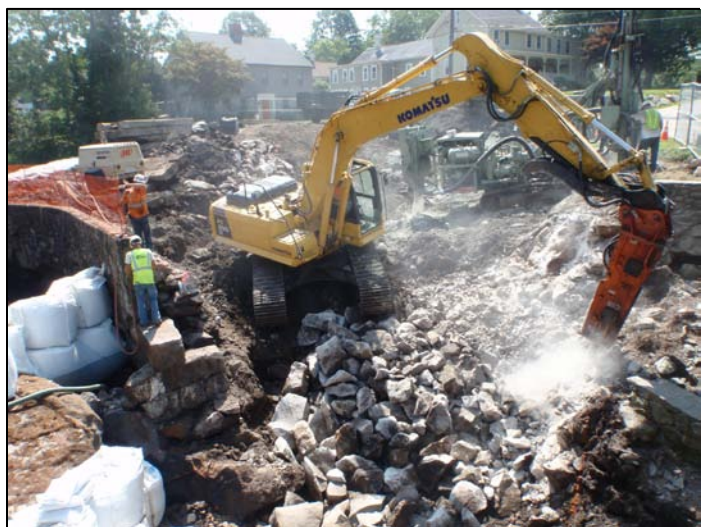
Construction at the Horseshoe Falls Dam. Photo by Jim Turek , IMSG/NOAA Restoration Center.
